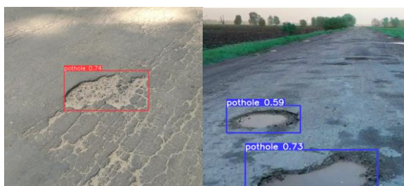
Fig:5 Output of images and video showing pothole
